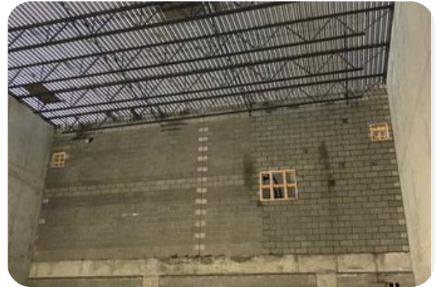
Gym block wall
