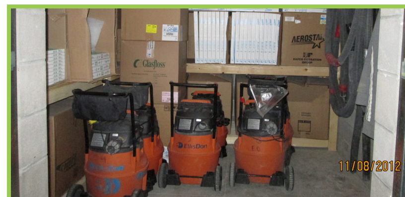
Keeping construction site clean and using vacuums with HEPA filter for clean up.
