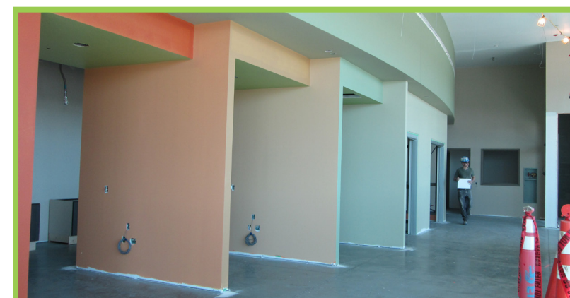
Sequencing construction activities so that carpets are installed after painting is complete.
